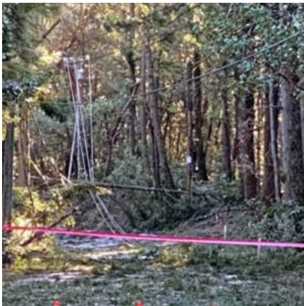
Close-up of downed power lines
