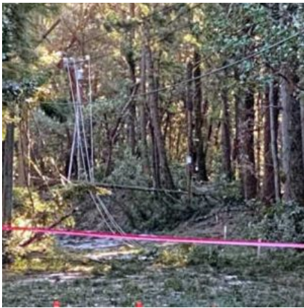
Close-up of downed power lines
